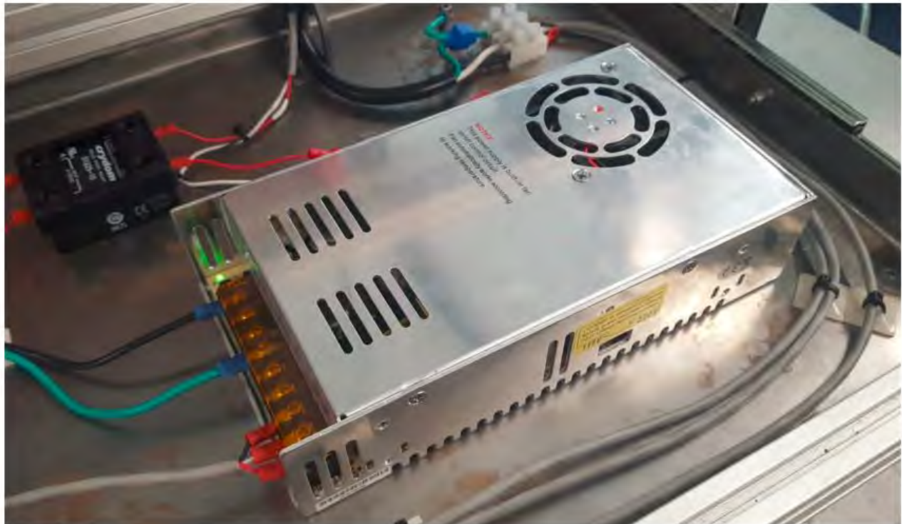
Figure 31 - S-400-24 Power Supply Installed in Prototype
