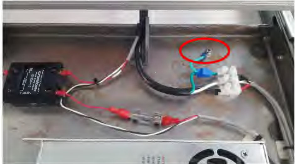
Figure 42 - Location of System Earth Ground (Circled in Red)
