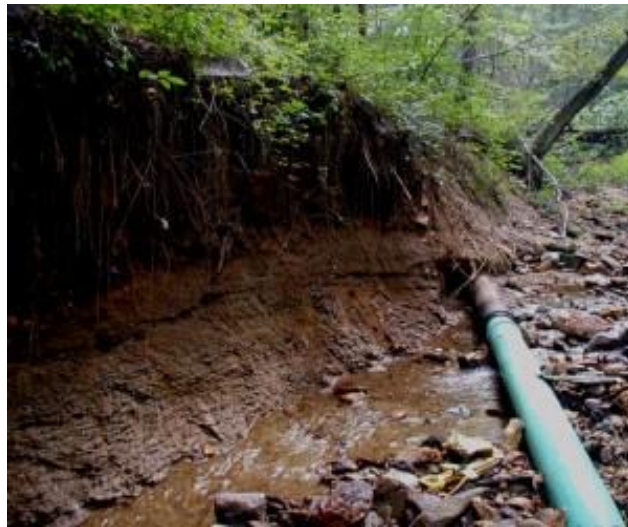
Figure 11 : Stream Bank Erosion (Arlington, 2015)
