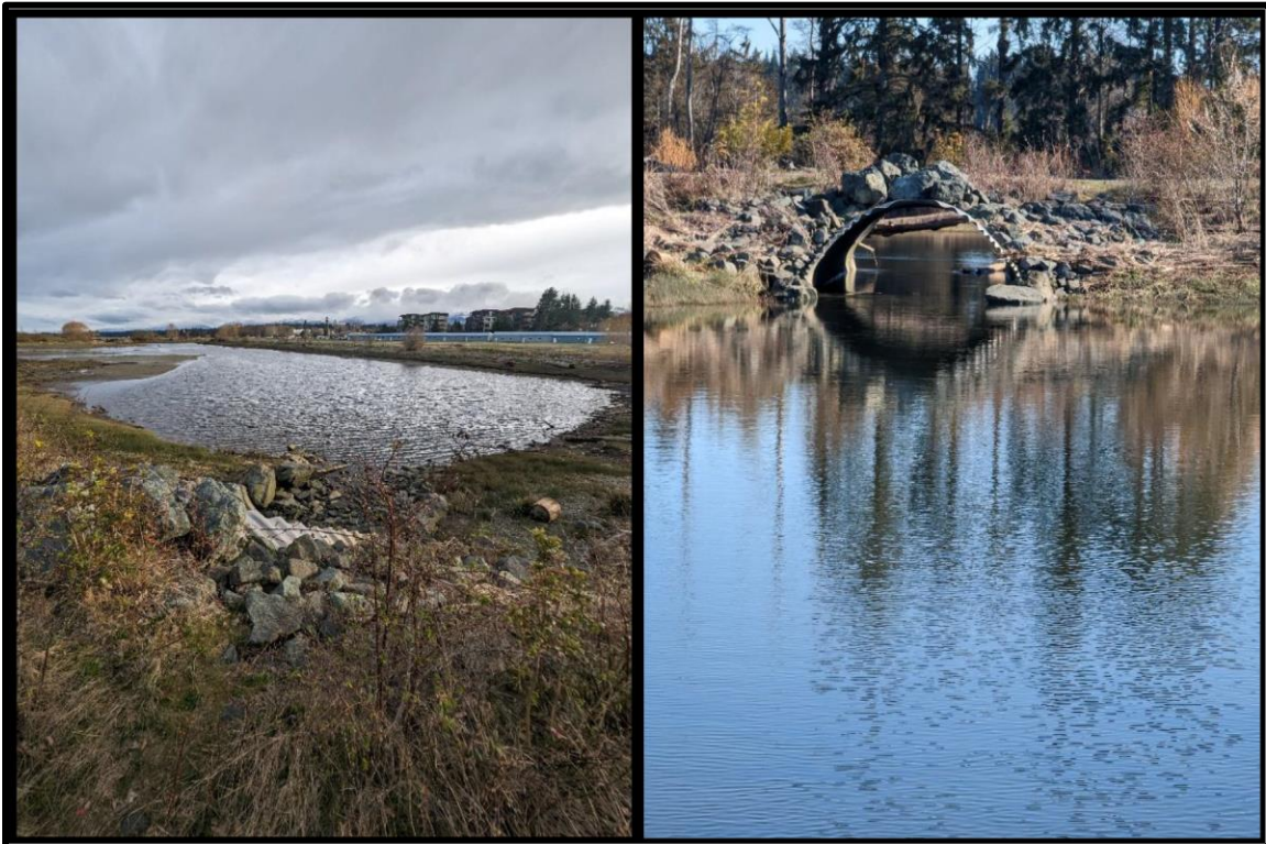
Figure 2: Airpark Lagoon restoration site. Photo of the lagoon from the north end of the lagoon facing south (left), and photo of the culvert installed at the north end of the lagoon increasing connectivity and waterflow between the lagoon and the Courtenay River (right).
