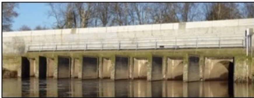
Figure 4: Elgin road sea dam on Nicomekl River west side, Surrey lowlands BC (JC Taft, 2016).
